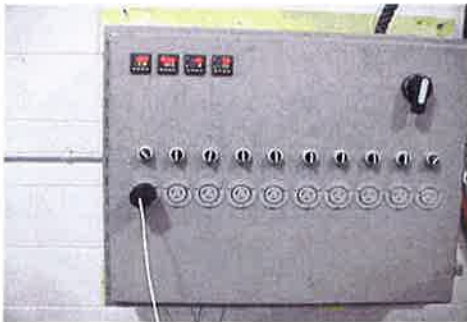
Control Panel with Ten Wand Connections and Four Controllers
