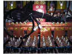
Power Supply Buss
